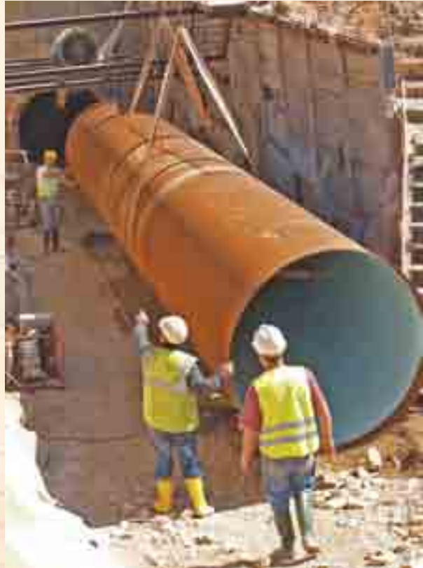
Doubling of the Castelo Bode trunk main between Quinta da Marquesa and the tower plant at Vila Franca de Xira
