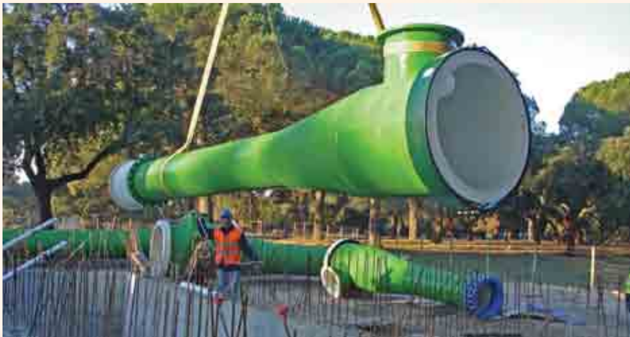
Macromasurement project for fighting water losses. Placement of flow meters.
