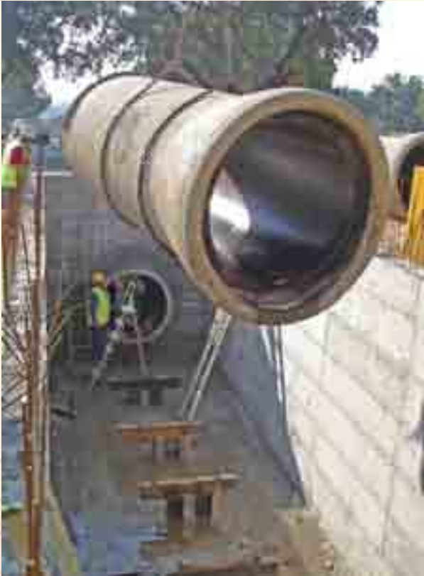
Macromasurement project for fighting water losses. Placement of flow meters in the tower mains at Vale da Pedra.
